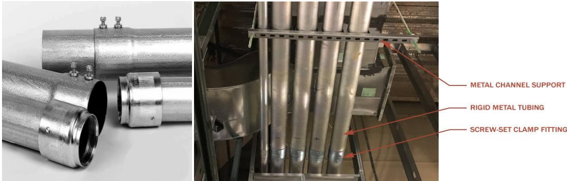
Figure 16. Electrical Metallic Tubing
