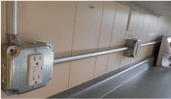
Figure 4. Conduit wall mounted
